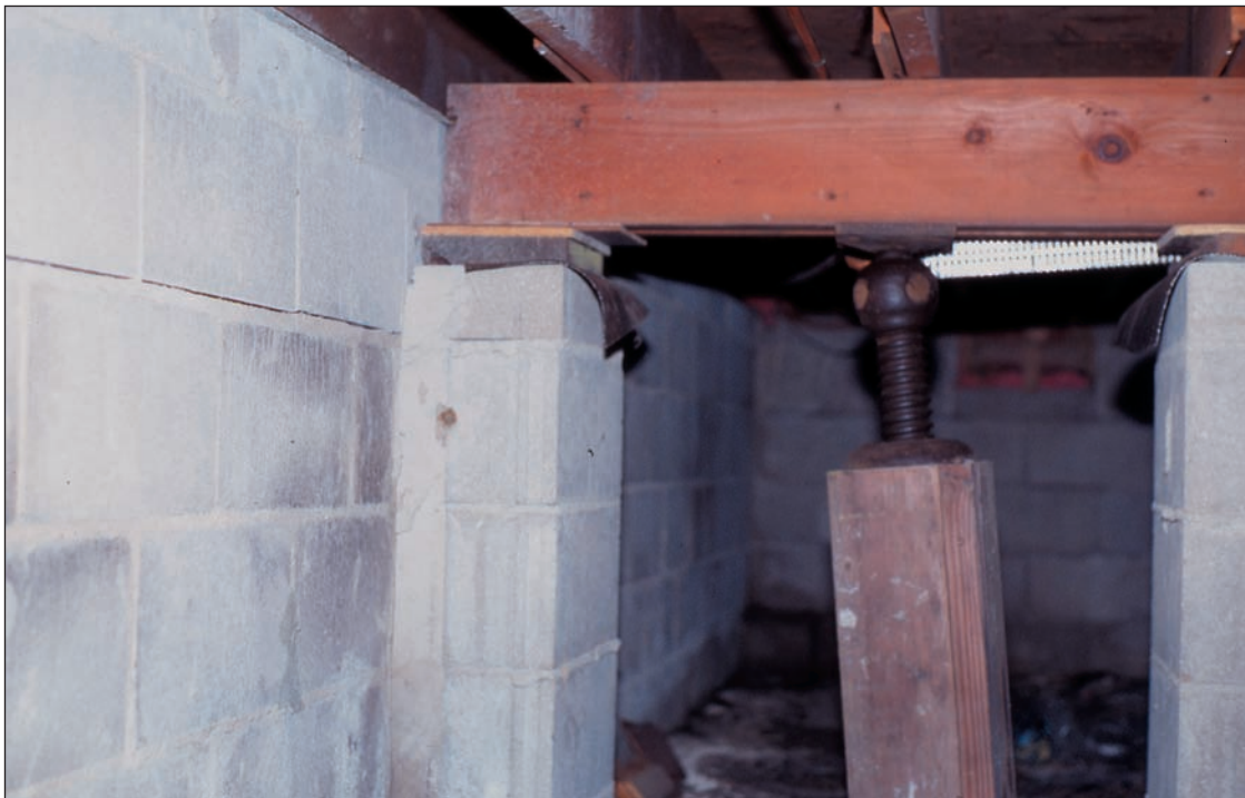
Figure 25 This main beam is not attached directly to the foundation wall. Because the beam is settling a different amount than the foundation and because some of the thick layers of shims are compressing, cracks have developed in the house above the beam.
