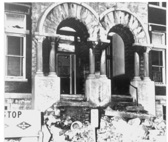
City building near Henderson, KY damaged by the November 9, 1968 earthquake.
