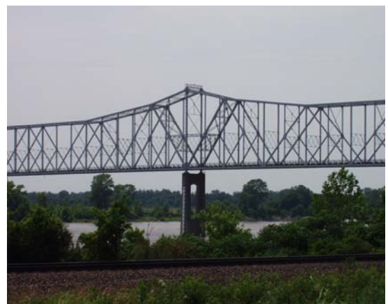
Chester Bridge – unprotected pier
