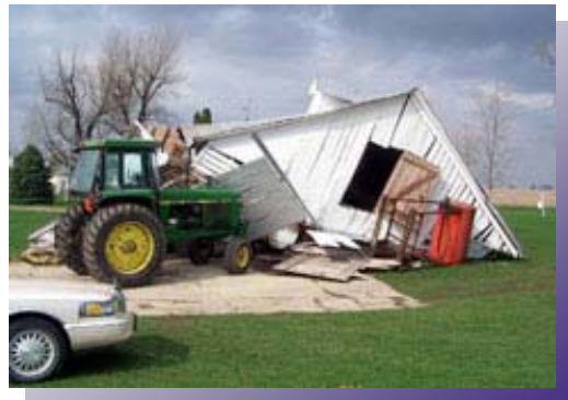
Damage sustained to a barn in rural Ogle County from a thunderstorm accompanied by high winds.
