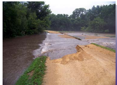
Recent flooding caused the Leaf River to overflow its banks and wash out a portion of White Eagle Road west of Adeline.
