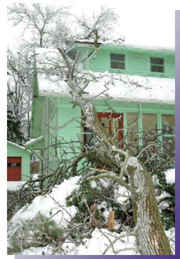
Damage sustained to a home in Mt. Morris during the December 24 th , 2009 ice storm.
