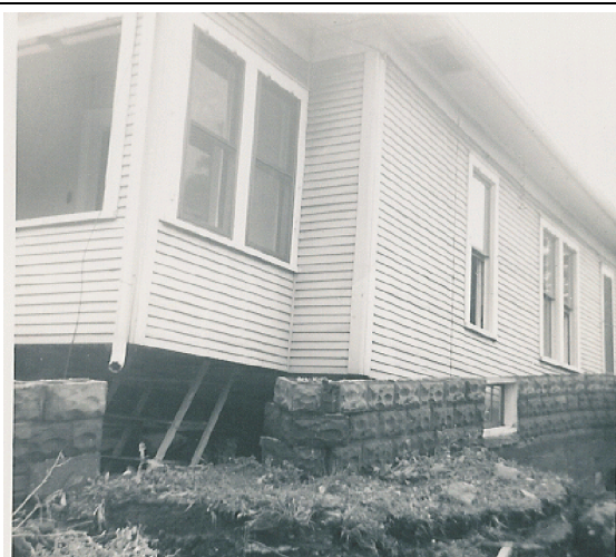
Soldier Creek flood damage, 1957
