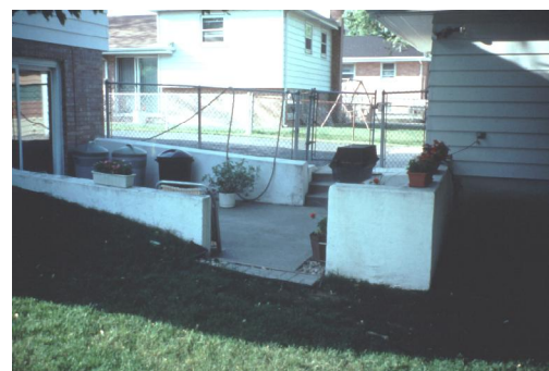
This floodwall in South Holland was installed after the owner attended a workshop on retrofitting. The community helped pay for the project with a rebate. It has kept floodwaters out of the house three times since it was built in 1991.
