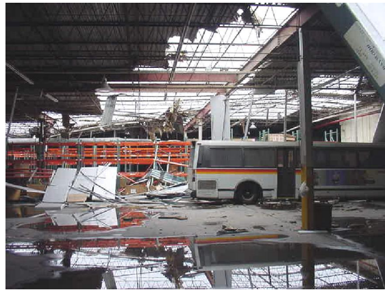
Damage from the April 2004 tornado
