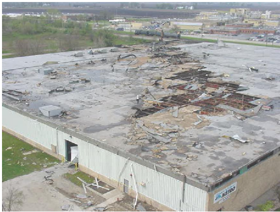
Damage from the April 2004 tornado
