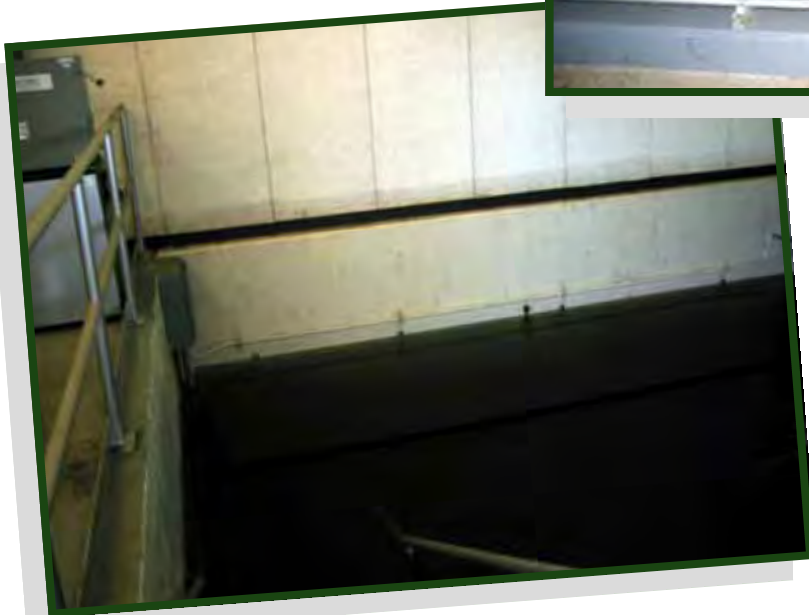
Flooding Inside Wastewater Treatment Facility
