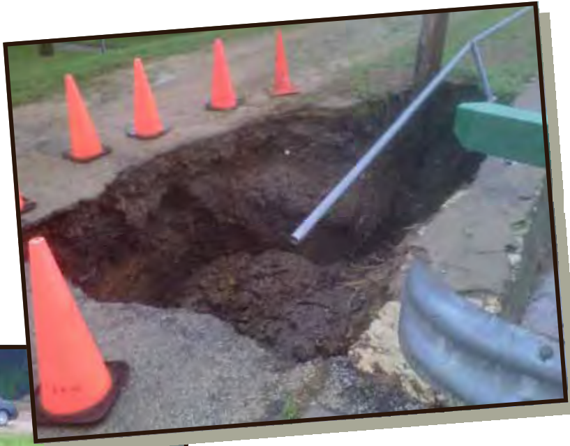
Flood damage to street
