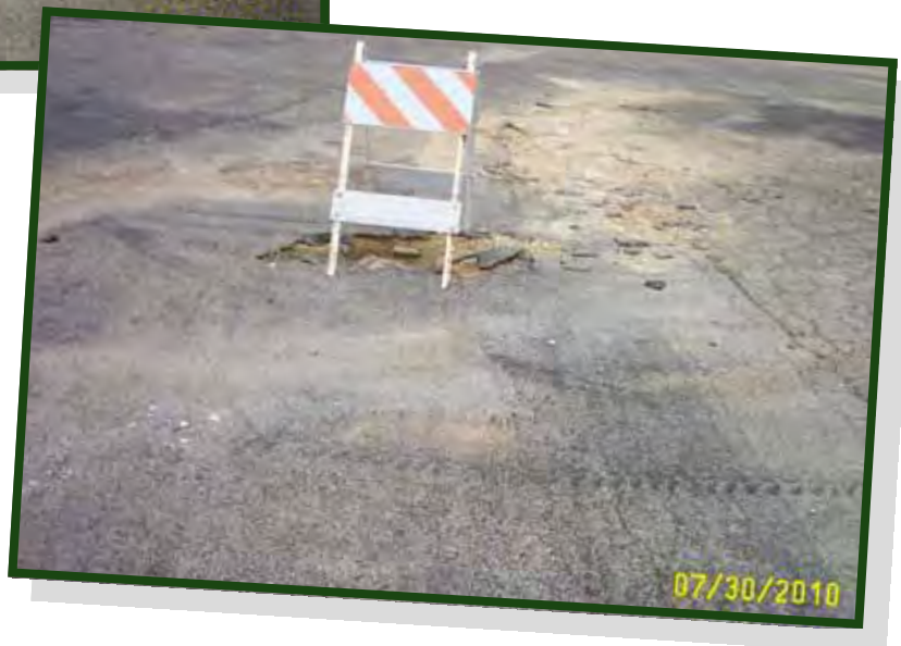
Roadway Damage Caused by Flooding
