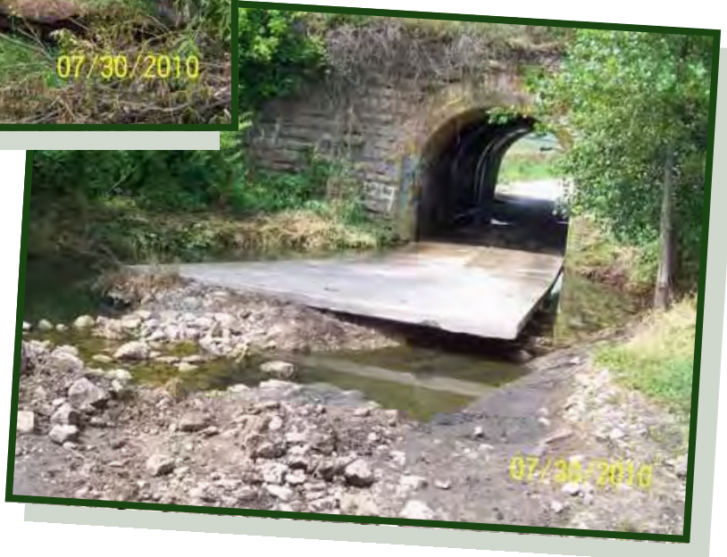
Flood Damage to Carr Road In Scales Mound Township
