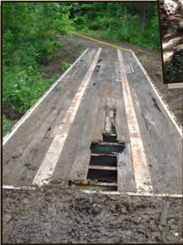
Bridge damage on Trail 5
