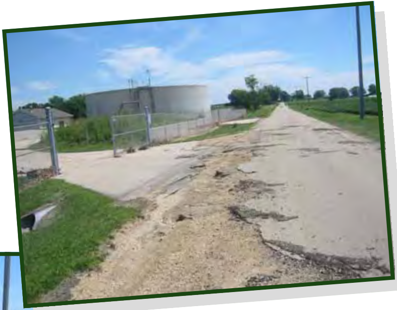
Roadway Damage in Front of Wastewater Treatment Facility
