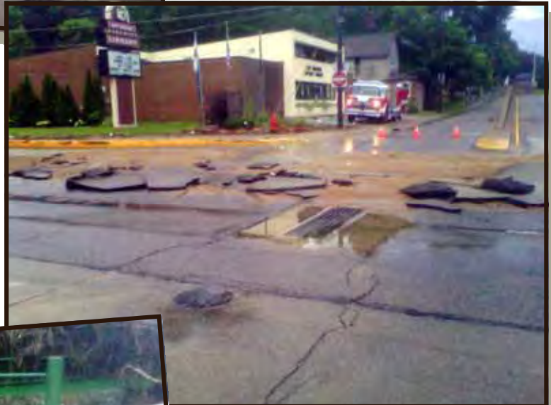
Flood damage to streets
