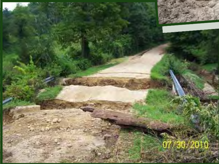
Flood Damage to Upman Road in Rush Township
