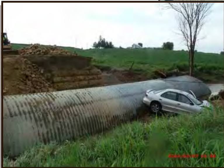
Flood damage to Chetlain Lane in Rawlins Township west of Galena
