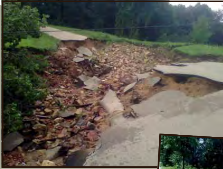
Flood damage to John F. Kennedy Road just west of East Dubuque
