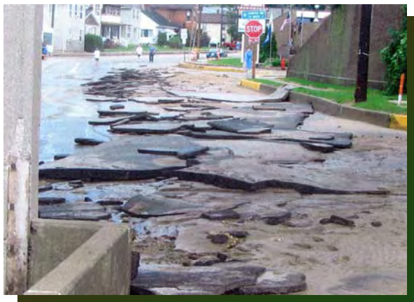
In East Dubuque, the force of flood waters from the July 2011 flash flood event broke up the pavement on several streets.
