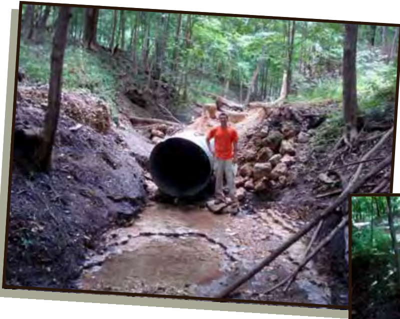
Flood damage to Trail 2 at Deer Hollow Creek
