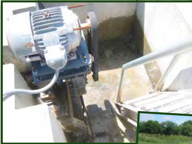
Flooding at Wastewater Treatment Facility
