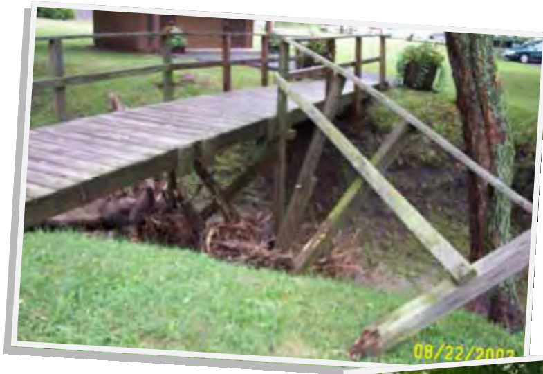
Marina Bridge Damage
