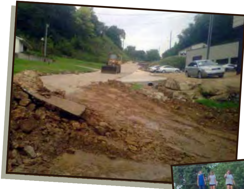
Flood damage to a roadway just outside of East Dubuque
