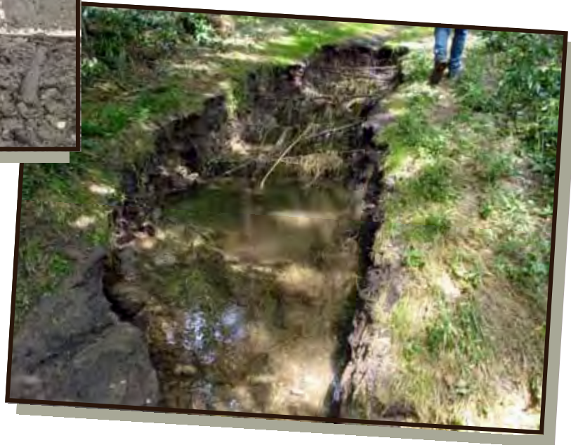
Flood damage to Trail 5 at Small Pox Creek
