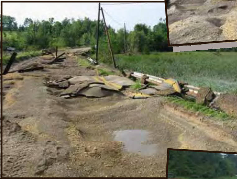
Flood damage to Blackjack Road
