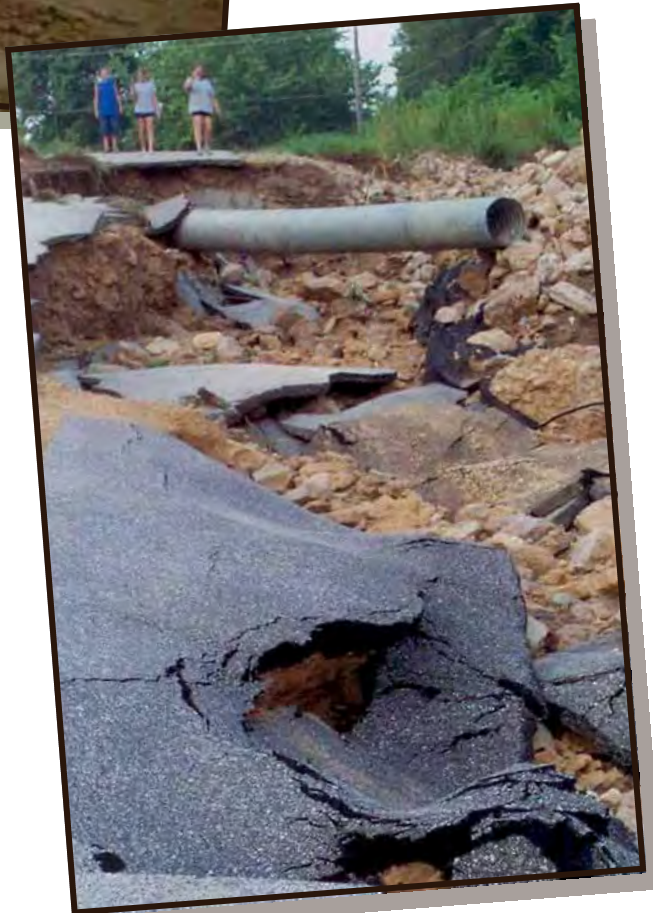
Flood damage to Tomahawk Lane just west of East Dubuque
