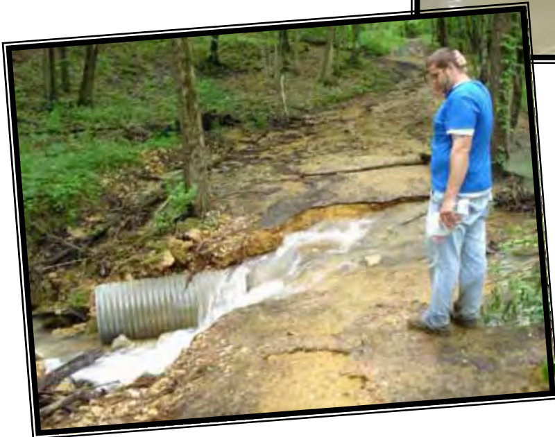
Damage to Trail at Belden School Lane
