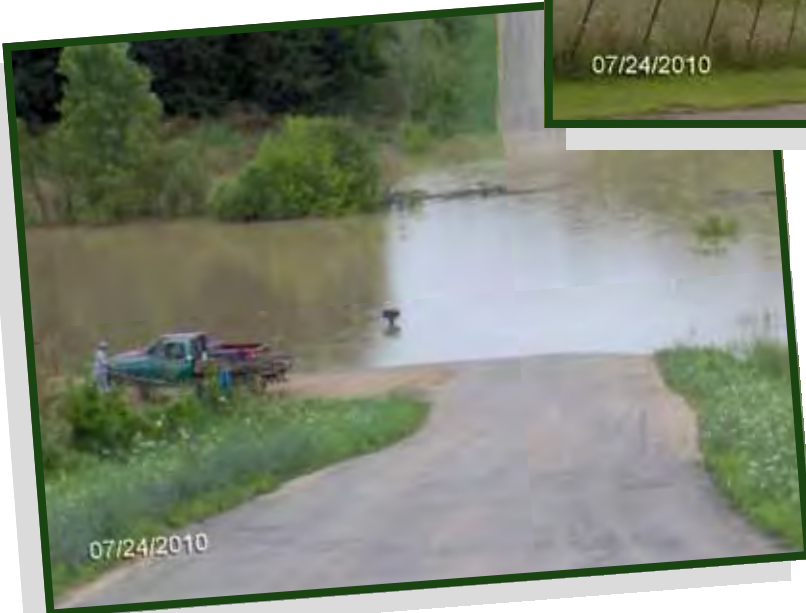
Roadway flooding in rural Jo Daviess County
