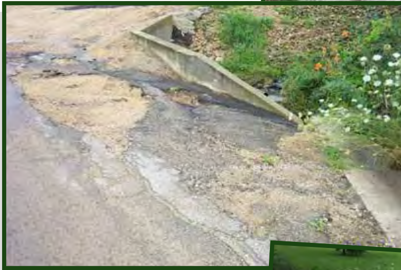
Roadway Damage Caused by Flooding
