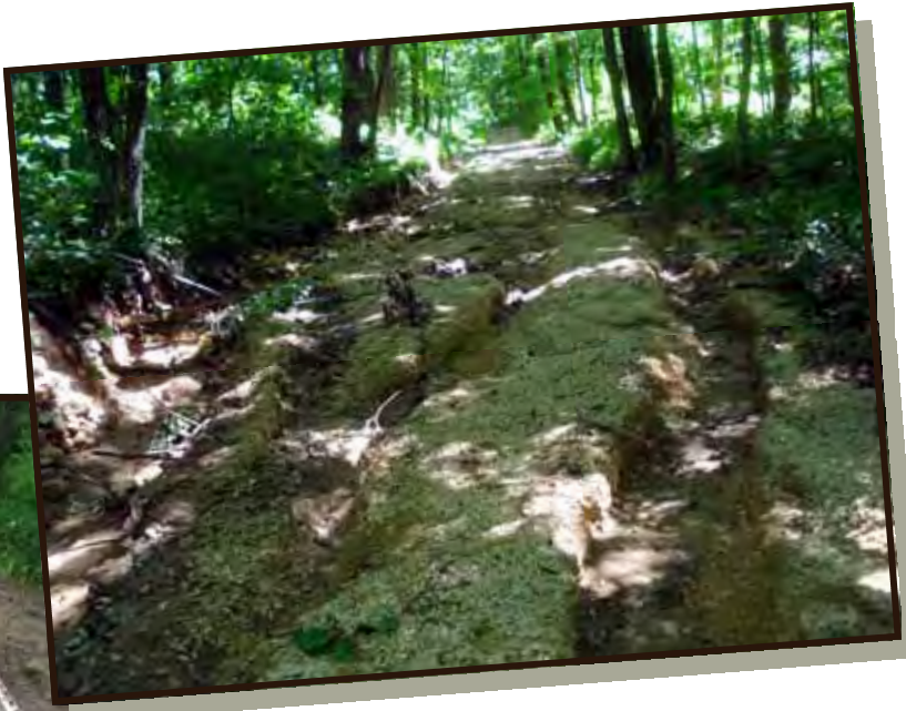
Flood damage to Trail 2B
