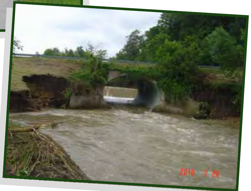
Flood Damage to Territory Drive
