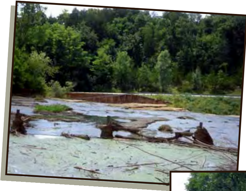
Flood damage to Thunder Bay Road taken from Lake Galena looking southwest
