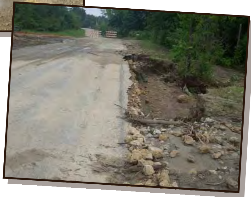
Flood damage to Blackjack Road near the Bautsch-Gray Mine in Rice Township southeast of Galena
