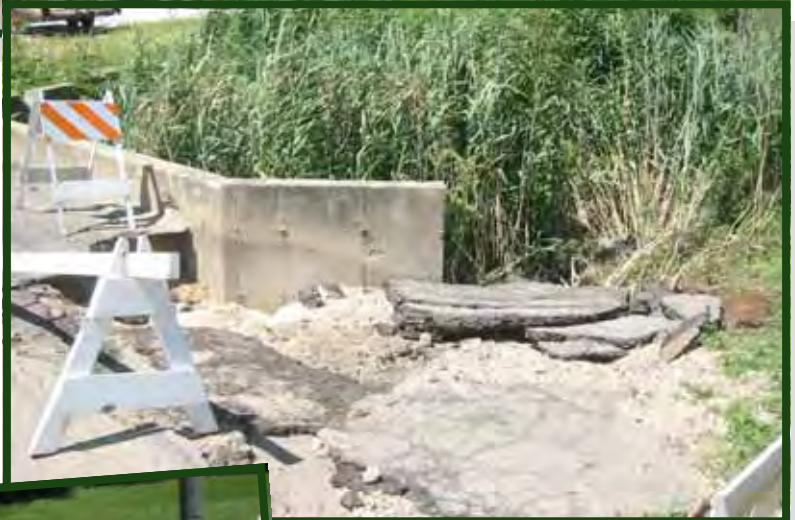
Roadway Damage Caused by Flooding
