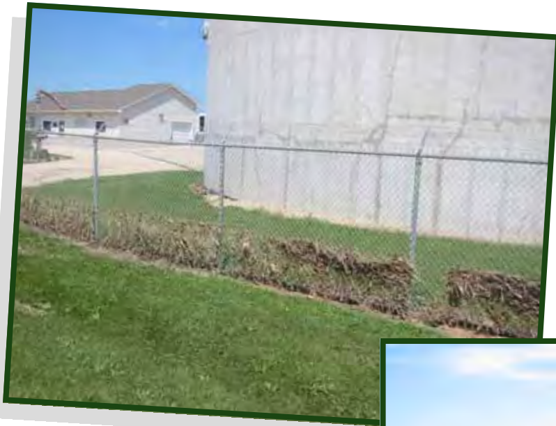
Debris Line from Flooding on Fence at Wastewater Treatment Facility
