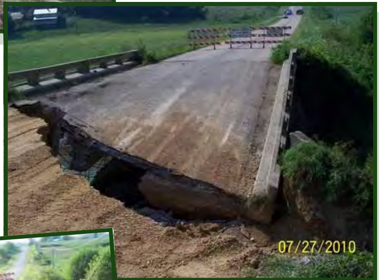
Flood damage to bridge on Bethel Road
