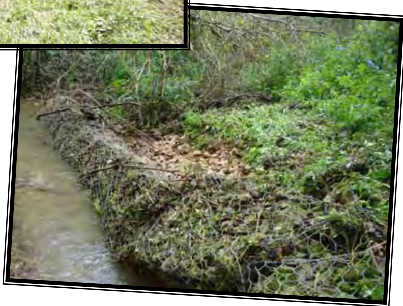
Gabion Baskets Undercut Along Trail 6
