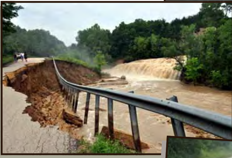
Flood damage to Thunder Bay Road near the Lake Galena Spillway
