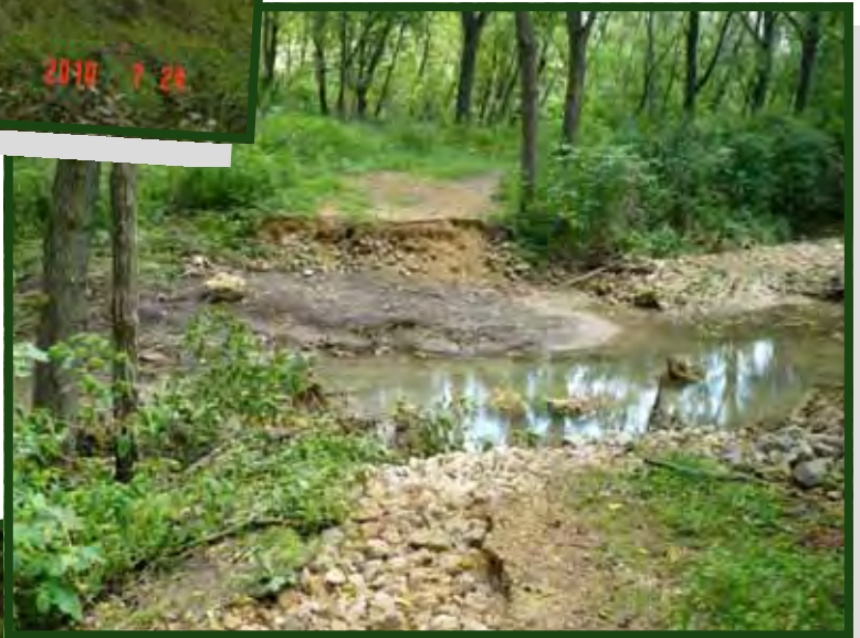
Flood Damage at Powderhorn Gap- Heatherdowns Lane Trail Crossing
