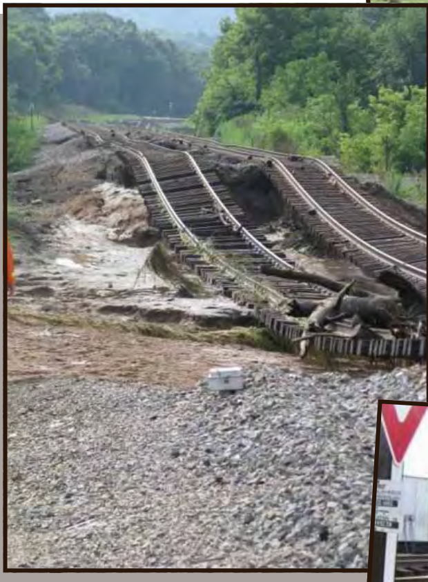
Flood damage to BNSF railroad tracks along South River Road in Rice Township near Aiken
