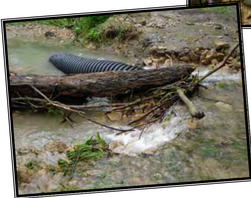
Damage on Trail 6A
