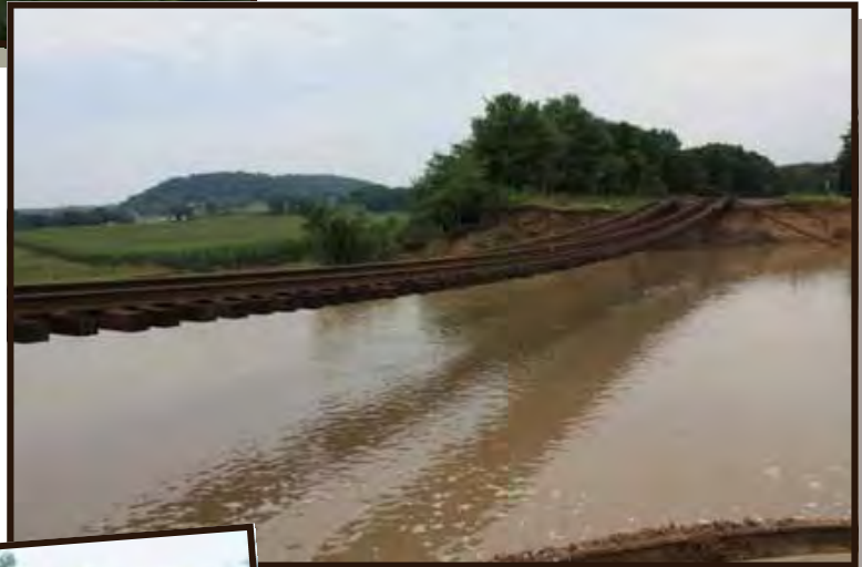
Flood damage to BNSF railroad tracks along South River Road in Rice Township near Aiken
