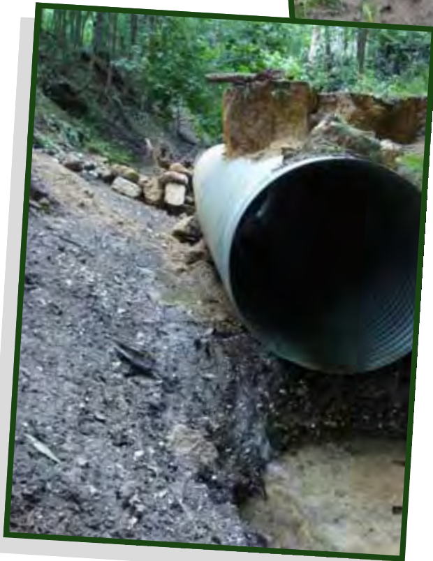
Flood Damage at Intersection of Trails 2 and 4
