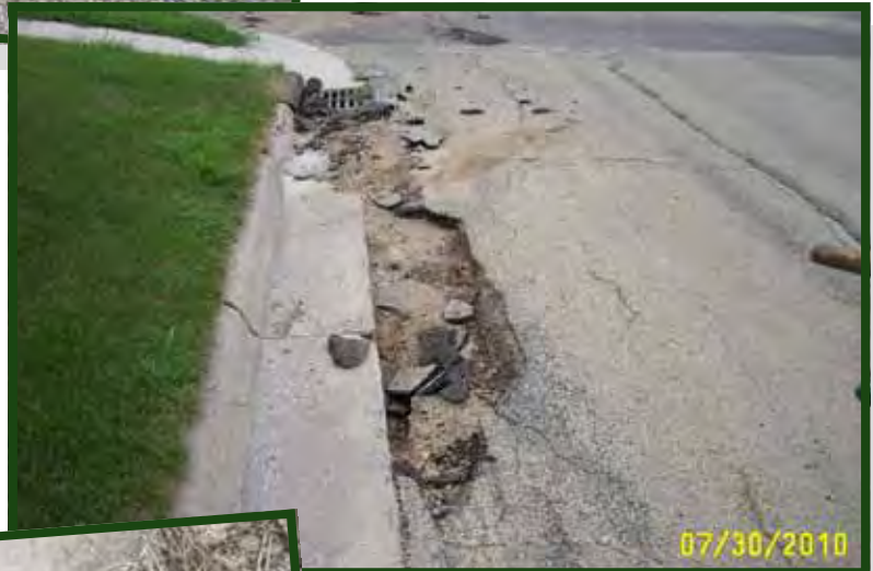
Roadway Damage Caused by Flooding
