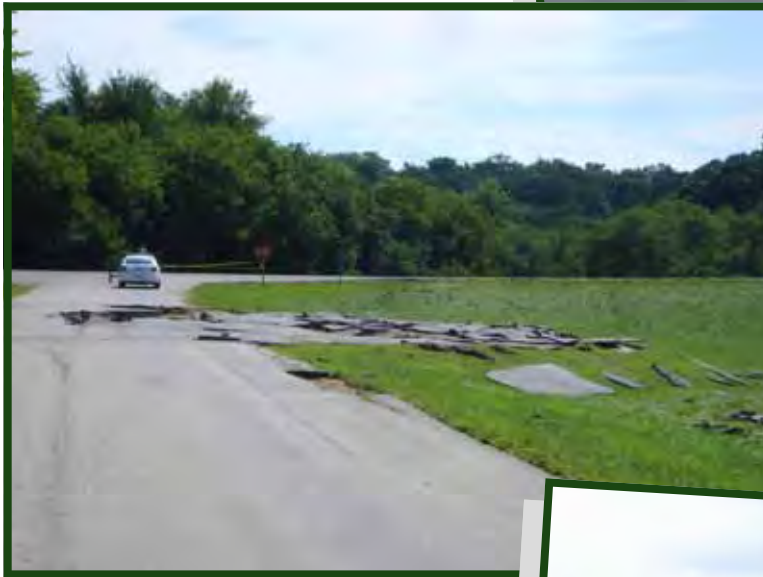
Flood Damage to Marina Drive
