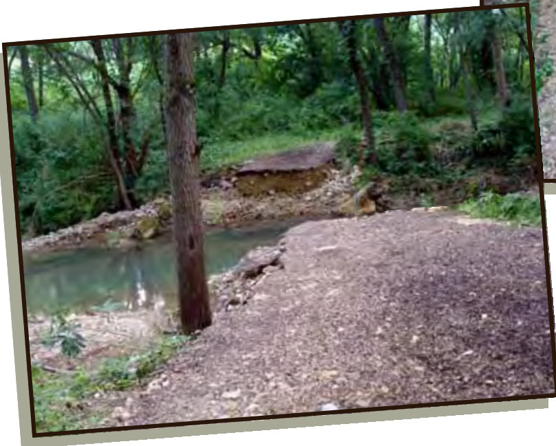
Trail 2 crossing washout
