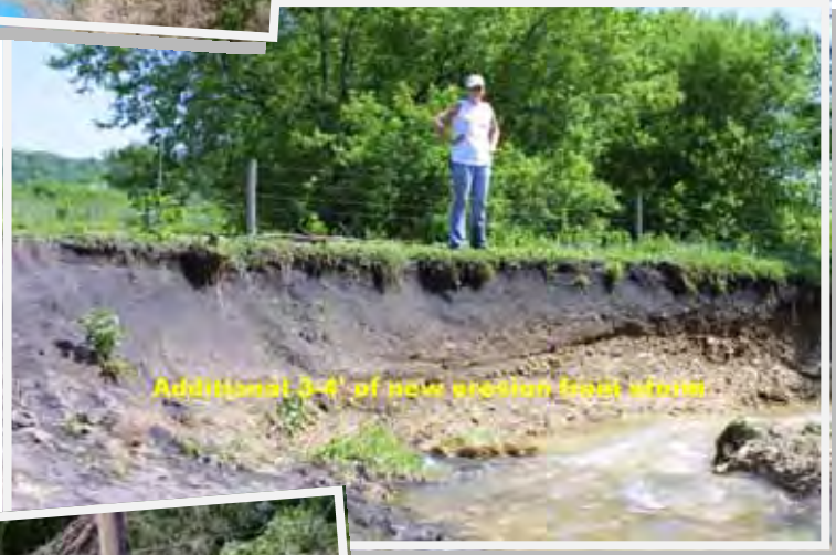
Shenandoah Riding Center Erosion
