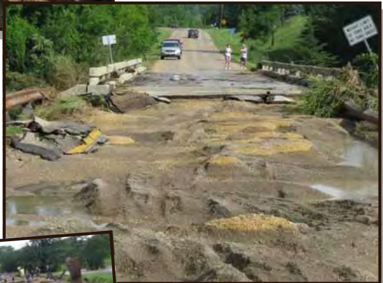
Flood damage to Blackjack Road near Small Pox Creek in Rice Township southeast of Galena
