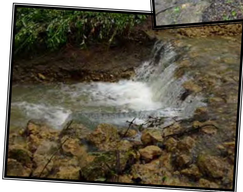
Washout on Trail 6A
