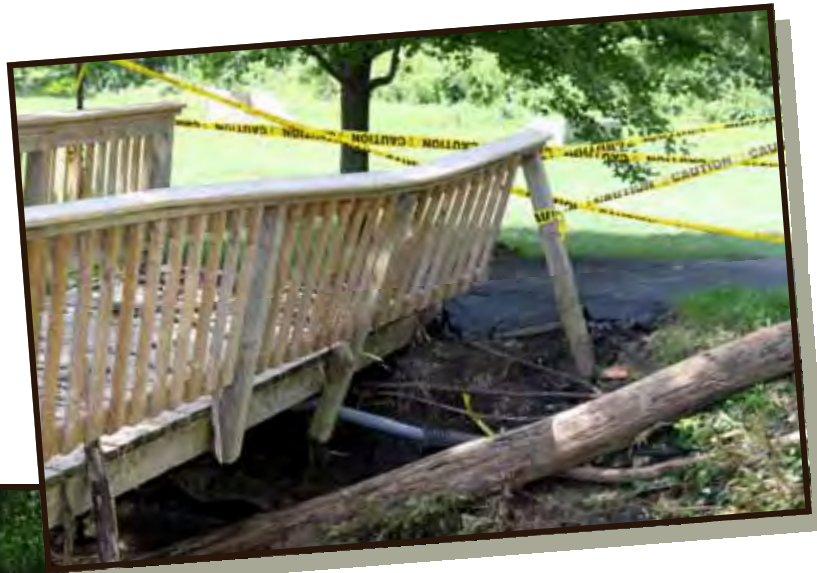
Damage to Marina Bridge
