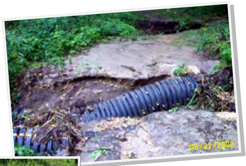
Trail Crossing Washout
