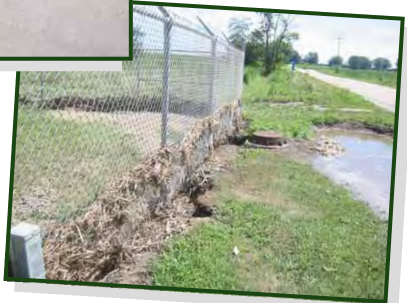
Debris Line from Flooding on Fence at Wastewater Treatment Facility
