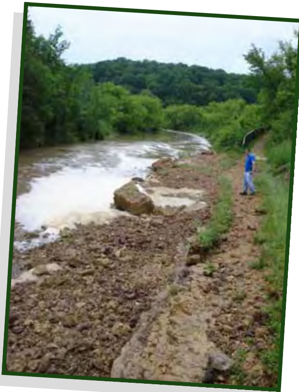
Flood Damage to Trail at Thunder Bay Falls Park
