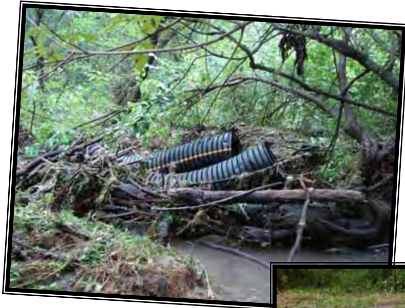
Damage to Trail 6 at No Name Creek
