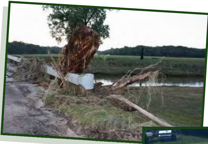
Debris lodged in guardrail along Apple River Road
