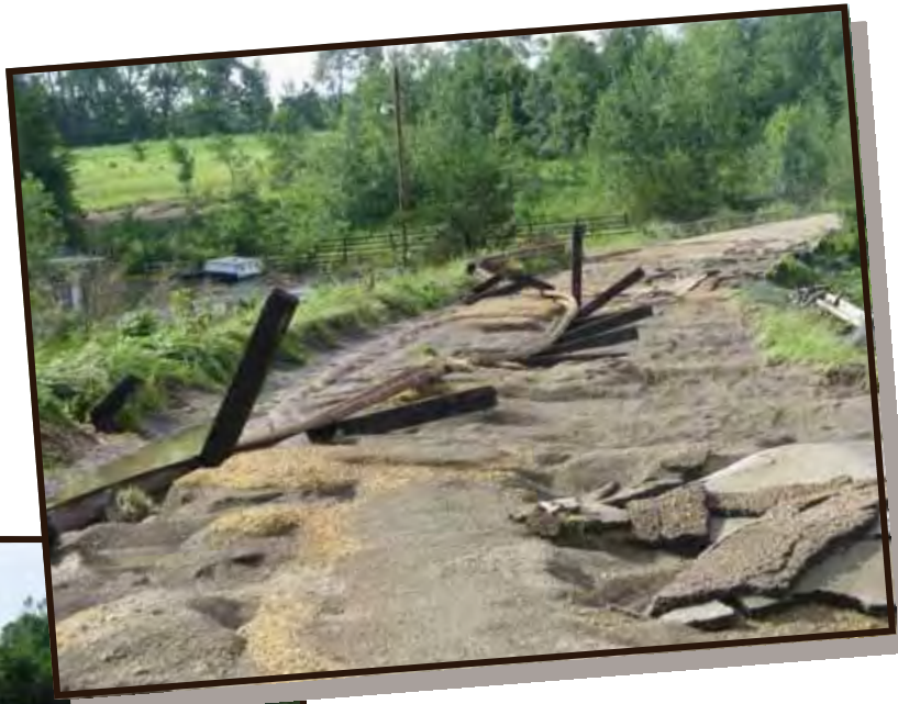
Flood damage to Blackjack Road near Small Pox Creek in Rice Township southeast of Galena
