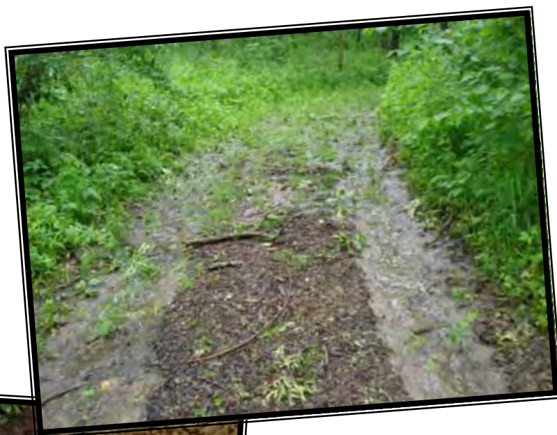
Flooding on Trail 6A
