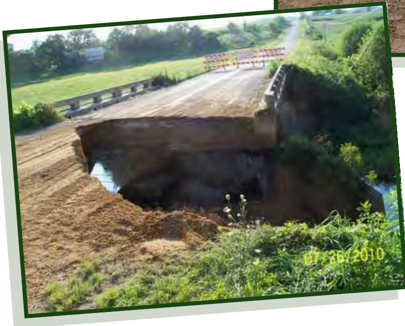
Flood damage to bridge on Bethel Road
