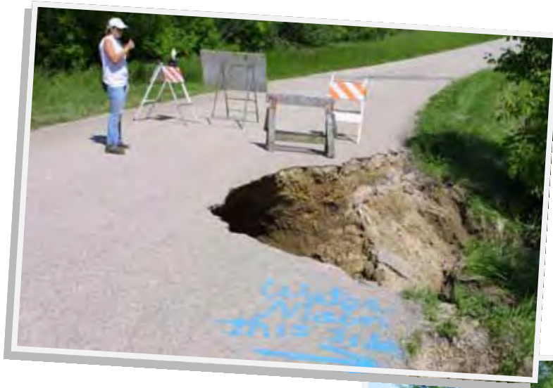
Shenandoah Drive Roadway Damage
