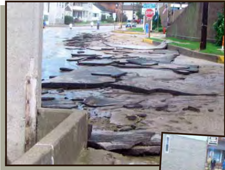
Flood waters broke up and undermined pavement
