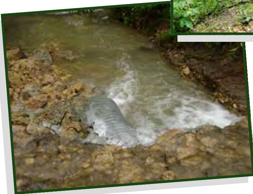
Culvert Overwhelmed by Water at Trail 6A
