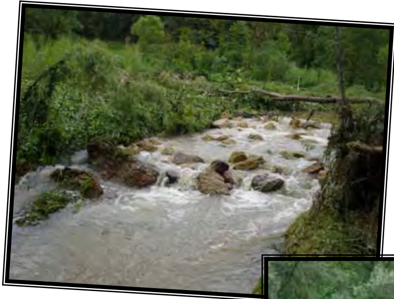
Weir Damage in North Cove
