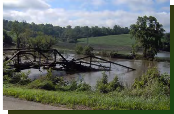
Portions of the Georgetown Road bridge were swept away during the flash flood event of July 2010.
