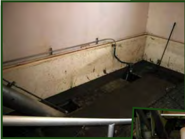
Flooding Inside Wastewater Treatment Facility
