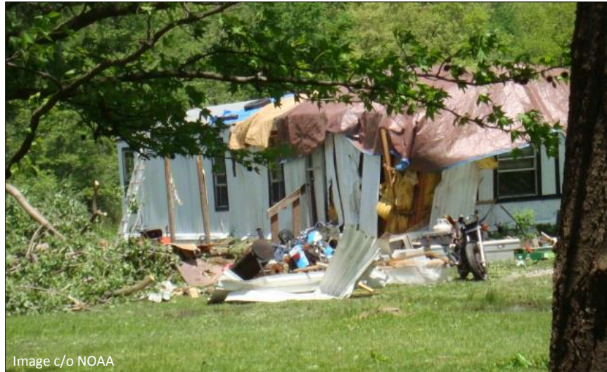
Figure 4-16. May 2009 Derecho - Damaged Mobile Home in Jackson County
