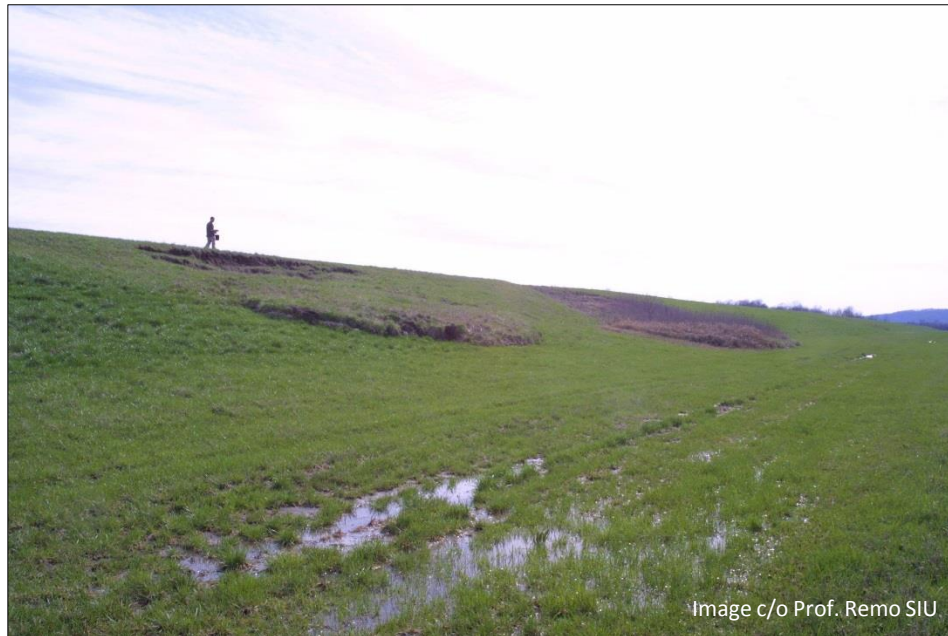
Figure 4-13. 2008 Slides along the Big Muddy Levee east of Grand Tower, IL
