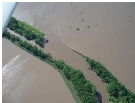
Levee breach along the Spoon River in mid-May 2009.
