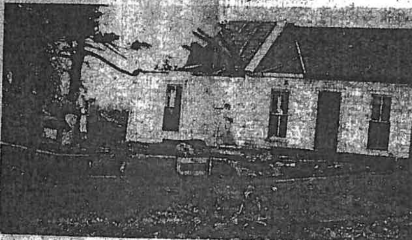
Neighbors survey the damage of the Bill Guymon farm home southwest of Loda today after a tornado Friday night ripped the house from its foundation and carried it 30 feet before setting it down. Mrs. Guymon and two children were injured and taken to Mattoon Memorial hospital. The tornado struck about 9:15 p. m. (Photo by Bertram Studio)
