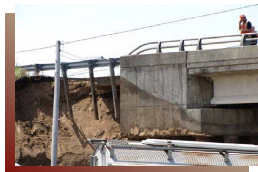
The Illinois 84 bridge over the rail lines was damaged by flood waters during the July, 2010 flash flood event.
