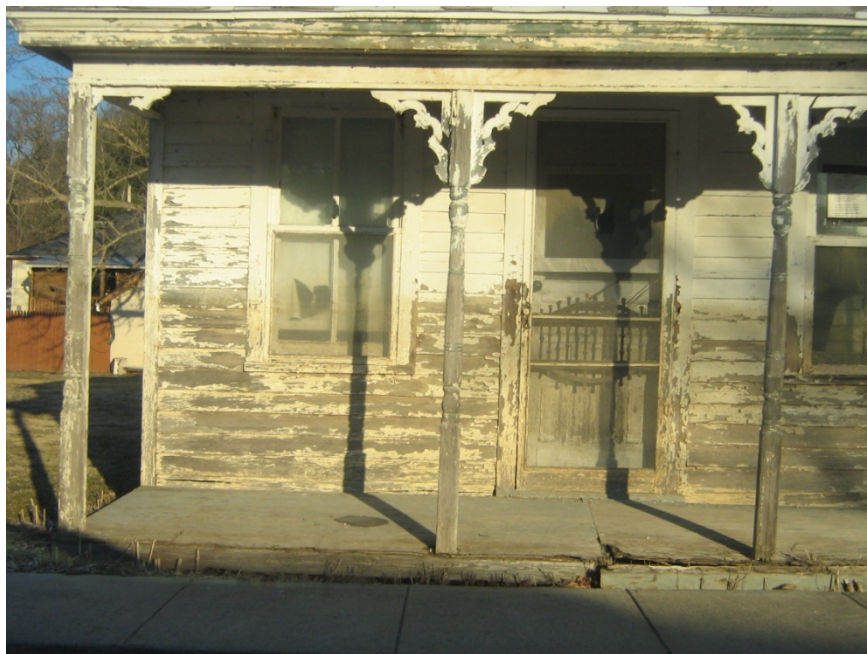
Figure 10. Home in Hamburg shows the high water mark from the 1997 flood.
