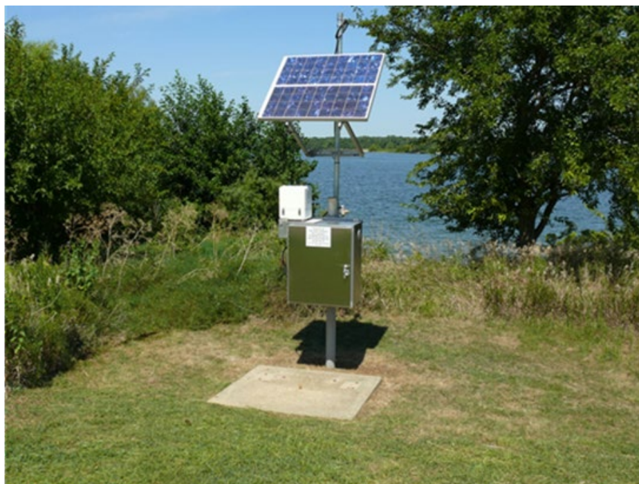
Figure 5. Typical IEMA-OHS GDN Field Installation
