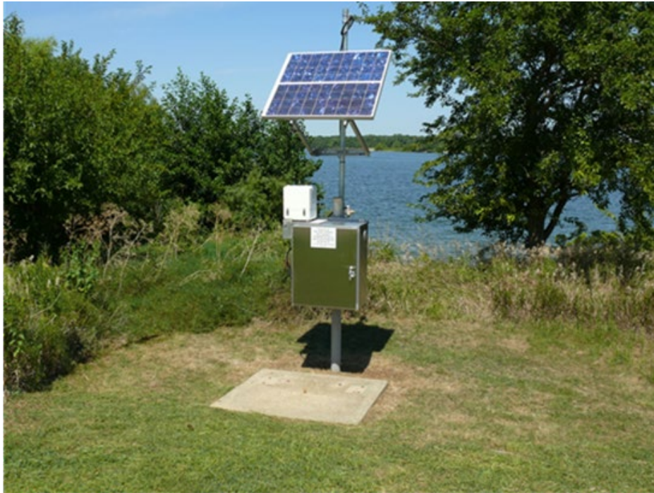
Figure 5. Typical IEMA-OHS GDN Field Installation
