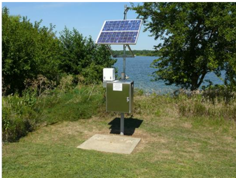
Figure 6. Typical IEMA GDN Field Installation
