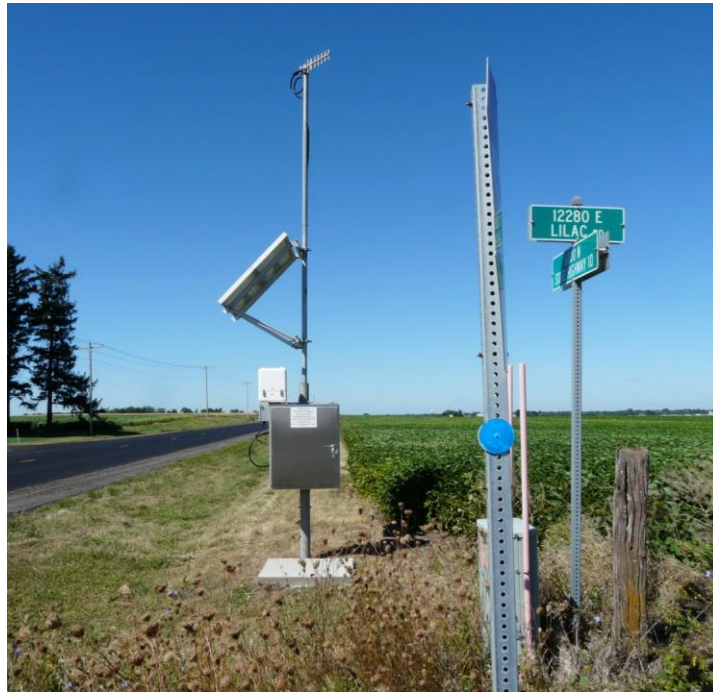
Figure 7. Typical IEMA GDN Field Installation
